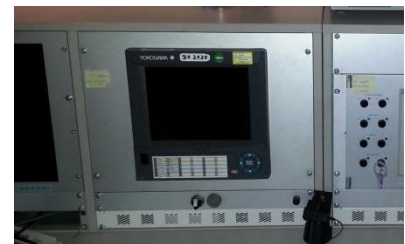
MV 100 built-in control room
